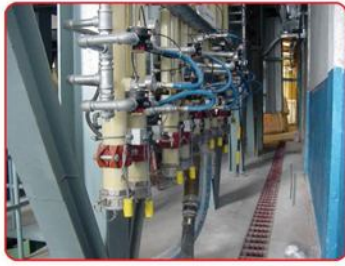
Manual Hose Switch for Silo Loading
