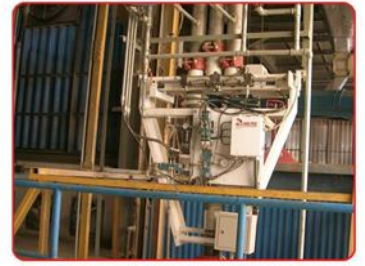
3 Way Diverter Switch for Animal Feed Factory
