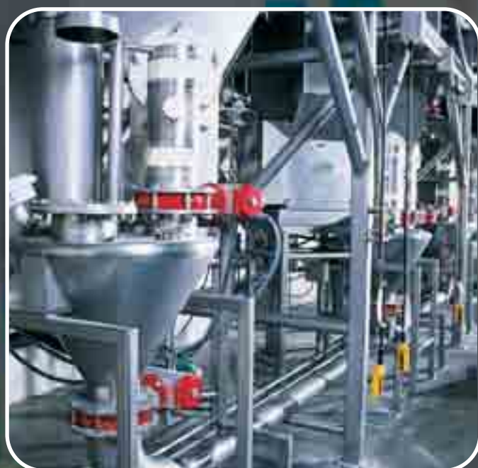
DENSE PHASE VACUUM INSTALLATION
